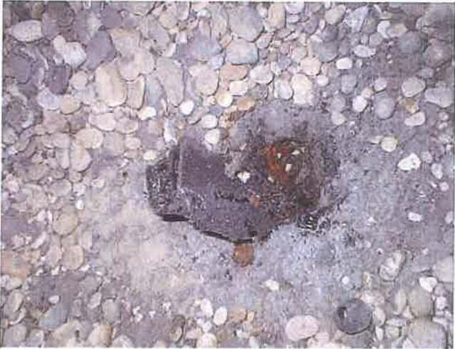
C) Area #5 Core Cut -Saturated Fiberboard Insulation
