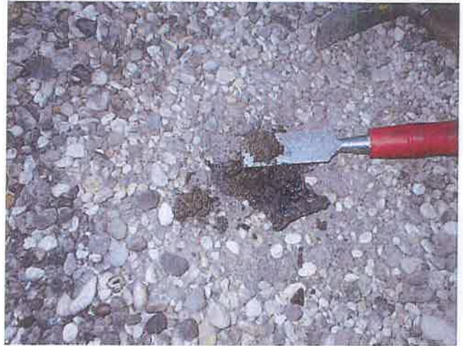
B) Area #2 Core Cut -Saturated Perlite Insulation
