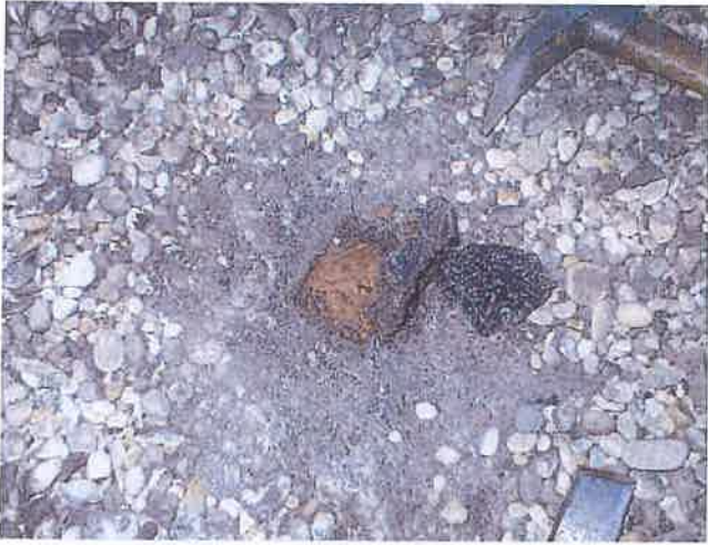
A) Area #1 Core Cut -Saturated Fiberboard Insulation
