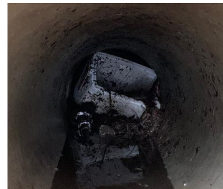
Coolers blocking Storm Pipes
