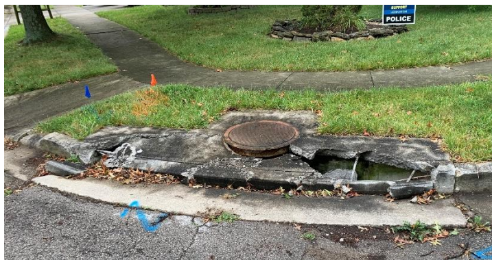
Completely Broken Inlets
