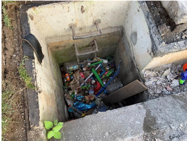
Curb Inlets full of Trash
