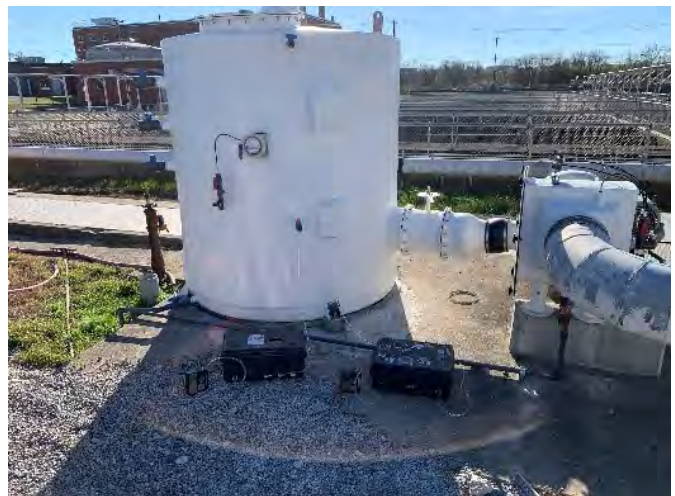
Odor Control System Testing Town Branch WWTP
