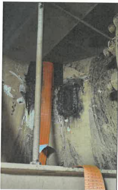
Figure 2: Existing damage/repair at elbow.
