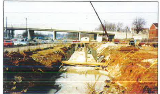
Chambered 12-foot x 6-foot storm and 5-foot x 4-foot sanitary R.C. Box Culvert - Downstream.
