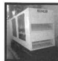
ON-SITE DIESEL GENERATOR
