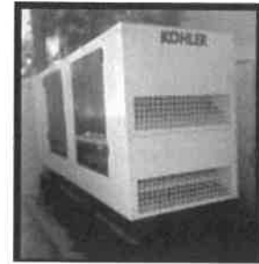
ON-SITE DIESEL GENERATOR
