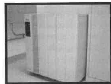
UNINTERRUPTIBLE POWER SUPPLY (UPS)
