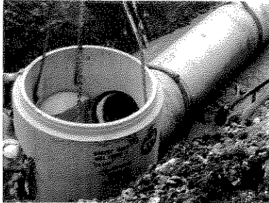
In 2012, Stantec designed approximately 22,600 LF of 36-inch and 48-inch sanitary trunk sewer for Nashville Metro.
