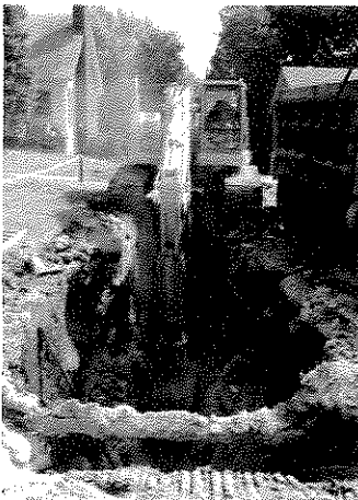
Stantec designed sanitary trunk sewer replacements for LFUCG in the approx. 40-year old Elkhorn Park neighborhood.
