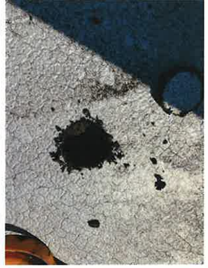
Cut Core Cut: Built up roof mopped right on top of the concrete deck. Water was sitting directly on the concrete deck showing that the roof has completely failed.
