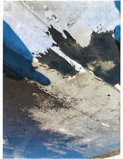
Close up view of how the ponding water has worn out his old roof over time. Multiple repairs have been made in this area to prevent water from entering the building.
