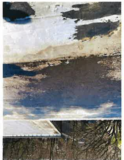
Ponding water that is deteriorated the Built-up roof over time.
