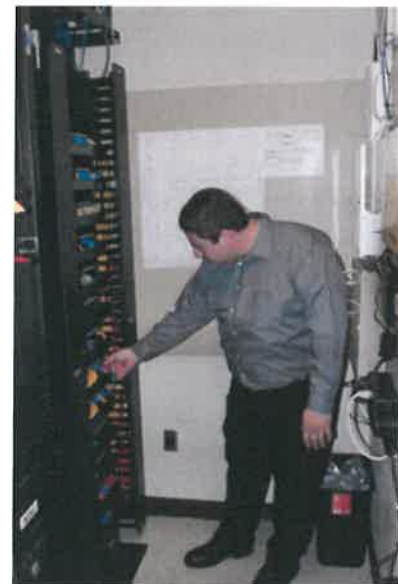
Comprehensive system testing is performed during both pre-staging and final system commissioning.
