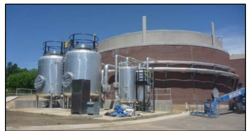
Dubuque anaerobic digesters and biogas conditioning.
