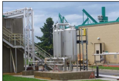
Biological H 2 S scrubbers.
