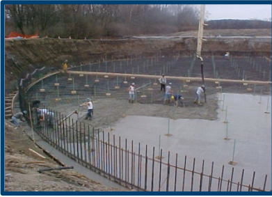
In 2010, B&N designed a 106 MG Equalization Basin for Louisville MSD. Stantec provided geotechnical engineering services on the basin.
