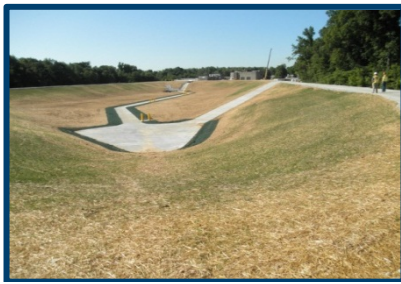
In 2011, Stantec designed the 20 MG Equalization Basin at the Guthrie WWTP
