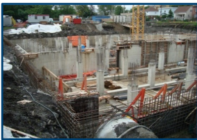
In 2007, Stantec designed a 4.4 MG below and above ground CSO storage facility for the City of Ottawa, Ontario that earned APWA's Project of the Year. The facility, located in Sandy Hill Park, was designed to maintain the character of the neighborhood by preserving community recreation and green space.
