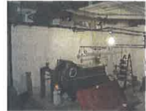
Septage Receiving Equipment - Columbus, IN
