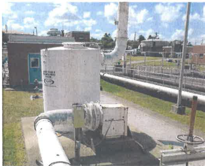
Scum Facility Odor Control System.
