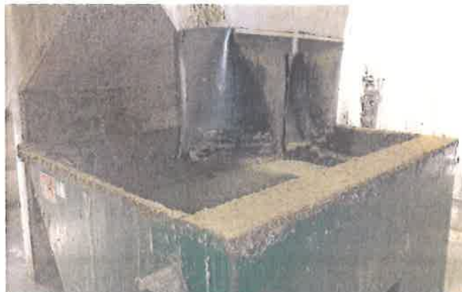
Scum Facility Discharge Chute and Hopper.
