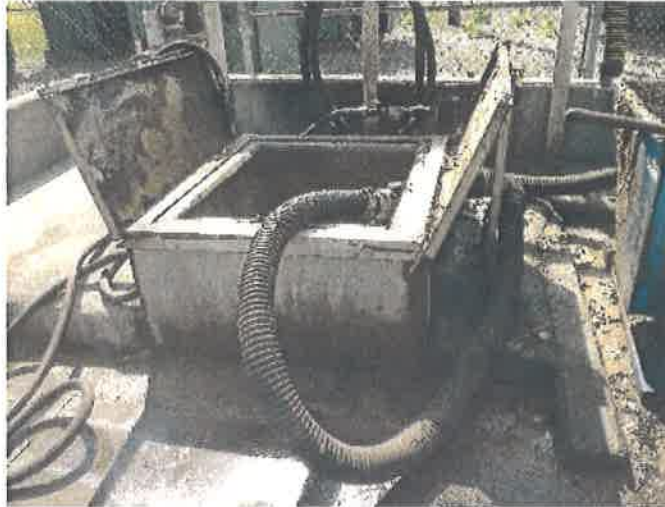
Existing Grease Receiving.
