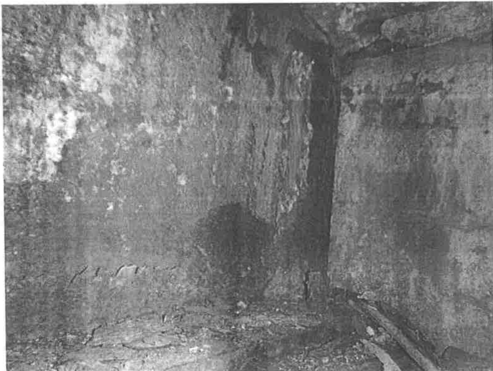
Beam end of beam #7 at abutment #2 has section loss in the last 3' of the beam
