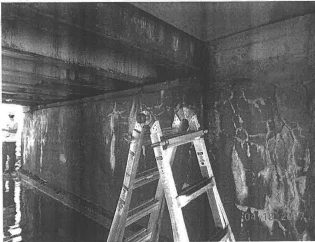
Cracking with efflorescence in the masonry coating on abutment #2
