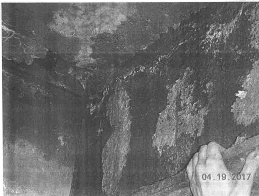
Beam end of beam #6 at abutment #1 has a 3"x2" hole in the web near the TF
