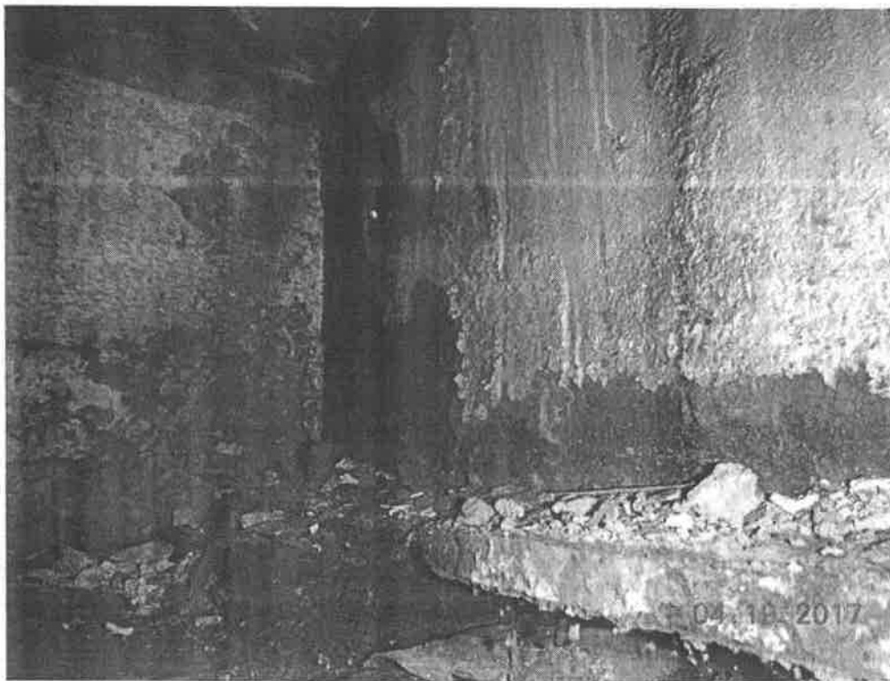
Beam end of beam #5 at abutment #2 moderate section loss in the web and LF with 1/16"-1/8" flange thickness.
