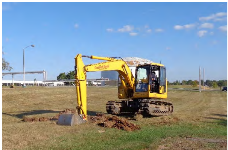
Ridgewater & Stantec advancing a test pit at the Lexmark Rainwater Harvesting System project in Lexington, KY.
