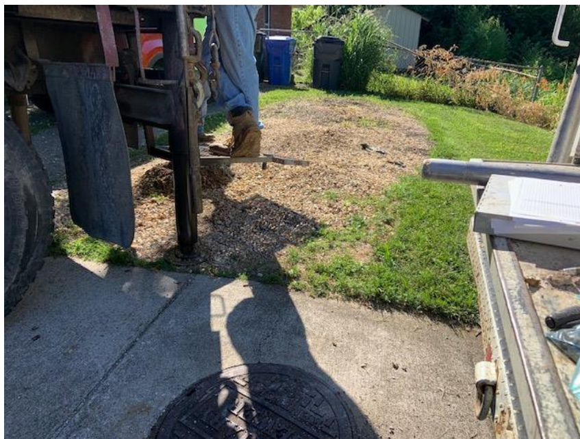
Figure 6: Crew working on drilling Boring B-3 on the east side of Crosby Drive and close to existing manhole MH-A23.
