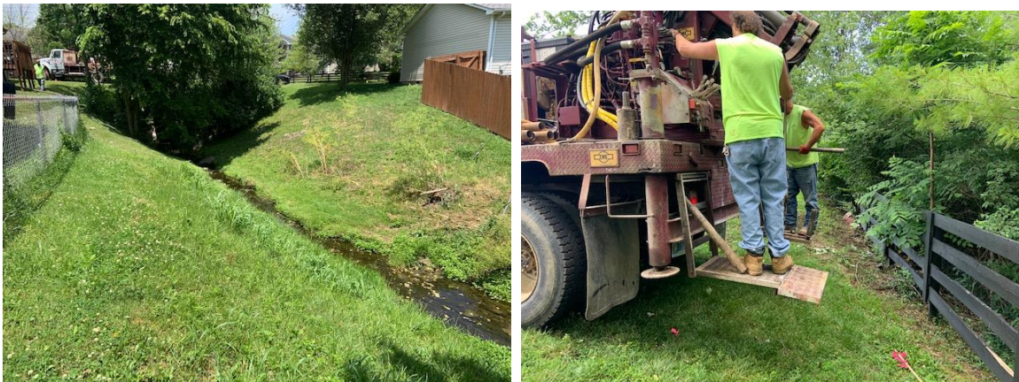
Figure 8 and 9: Crew working on drilling Boring B-1 (on the right). A view of the easement route and the creek on the east side of Appian way and close to Boring B-2.
