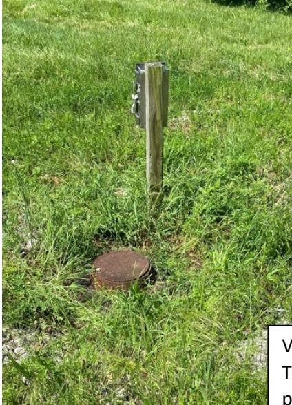
Ground surface view of augmentation well with electronic controls and water valve type access point.
