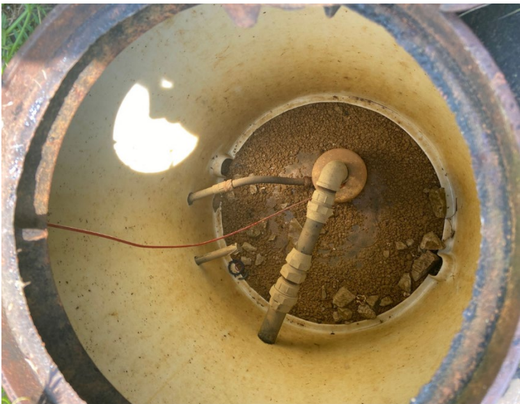
View inside the water valve access point at the top of the well head. This piping is approximately 2-3 feet below ground surface and is not easily accessible in this tight space.
