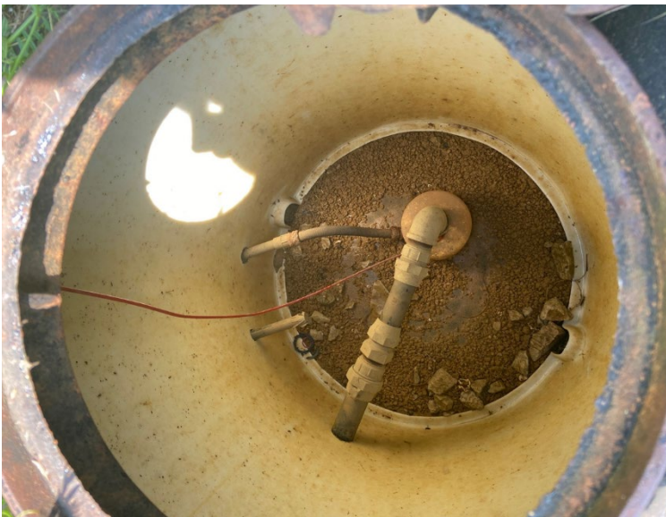
View inside the water valve access point at the top of the well head. This piping is approximately 2-3 feet below ground surface and is not easily accessible in this tight space.
