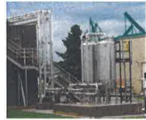
Biological H 2 S scrubbers.
