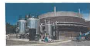
Dubuque anaerobic digesters and biogas
