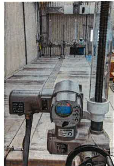
MRP UV Installation with modulating weir level control.
