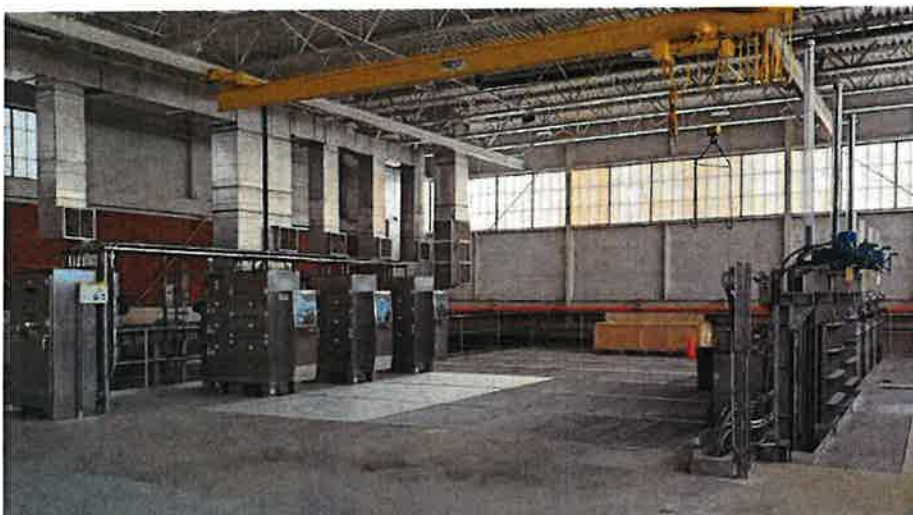
New Trojan UV Disinfection System – Madison Metropolitan Sewerage District.
