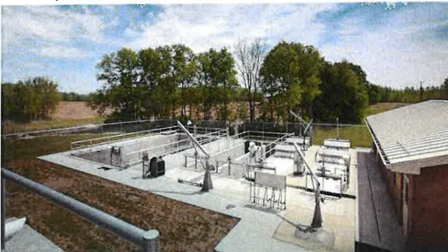
UV Disinfection Process at the CCU WWTF.
