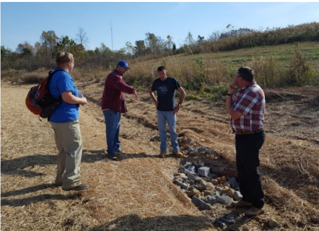
Casey Mattingly and Rain Storm meet on site with the owner and his construction supervisor to review the project
