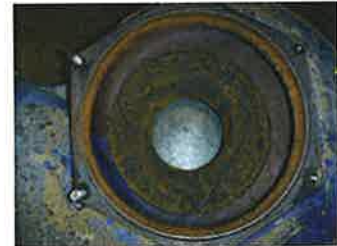
Inspection photo showing pitting on the existing dry weather pump impeller likely caused by vortices.
