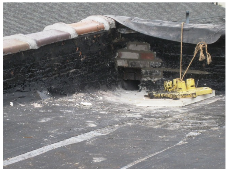
S. Corner: Roof is dried in with increased sump & slope to scupper.
