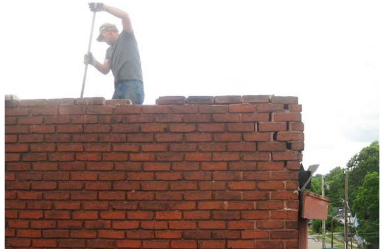
North corner of Roof Area 1: approx. 6' of clay tile copings came off during roof tear off
