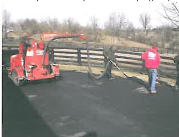
Crackfill “open cracks 1/4” & larger with hot rubber crackfiller with low pressure crackfill machine or “pot gravity drop”
