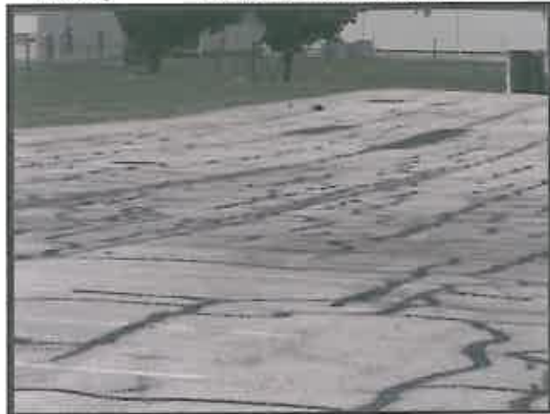
Parking lot with lots of Hot Rubber crackfill
