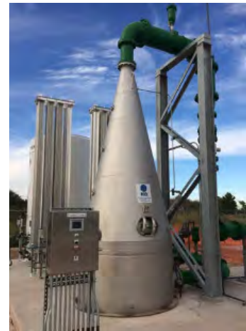
ECO2 superoxygenation system. Offers a high level of odor control in a compact footprint with relatively low yearly operations costs.
