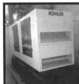
ON-SITE DIESEL GENERATOR
