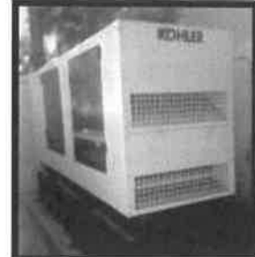
ON-SITE DIESEL GENERATOR
