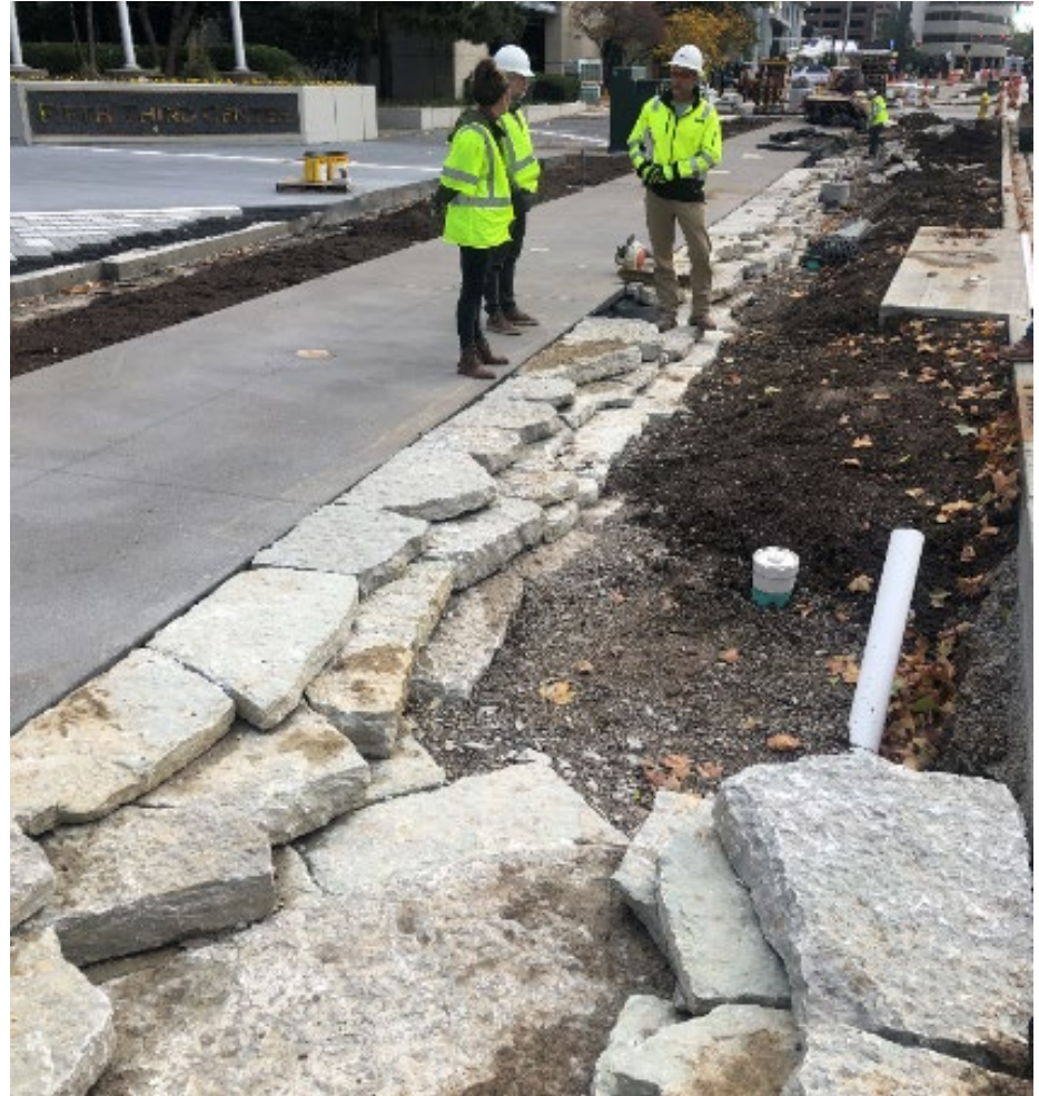
What looks like a normal plant bed above actually contains layers of drainage systems for storm water below.
