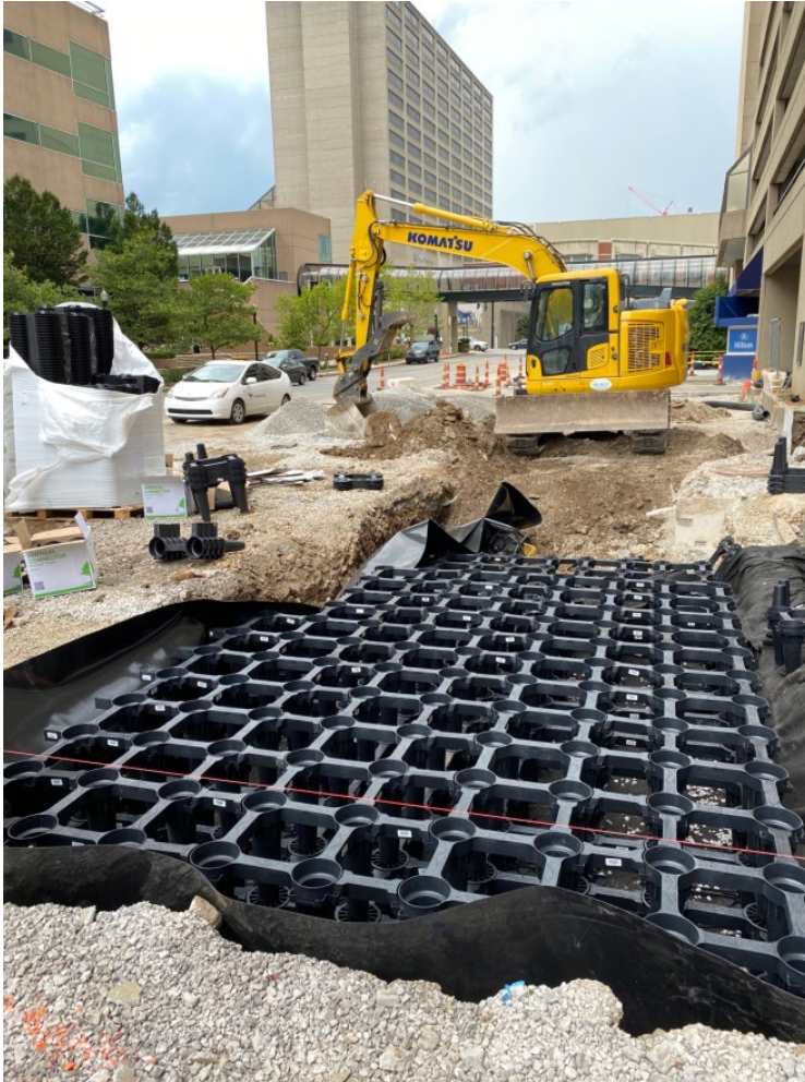
Soil cells are installed underground to provide a healthy environment for tree roots.
