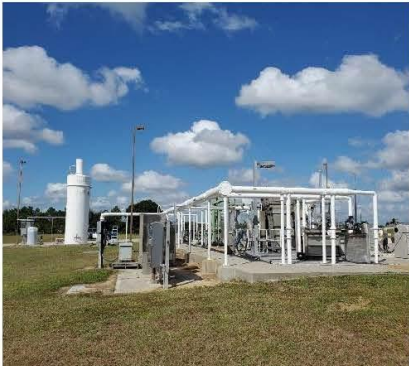
New Headworks Bioscrubber
