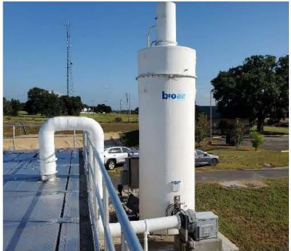
New Splitter Box Bioscrubber
