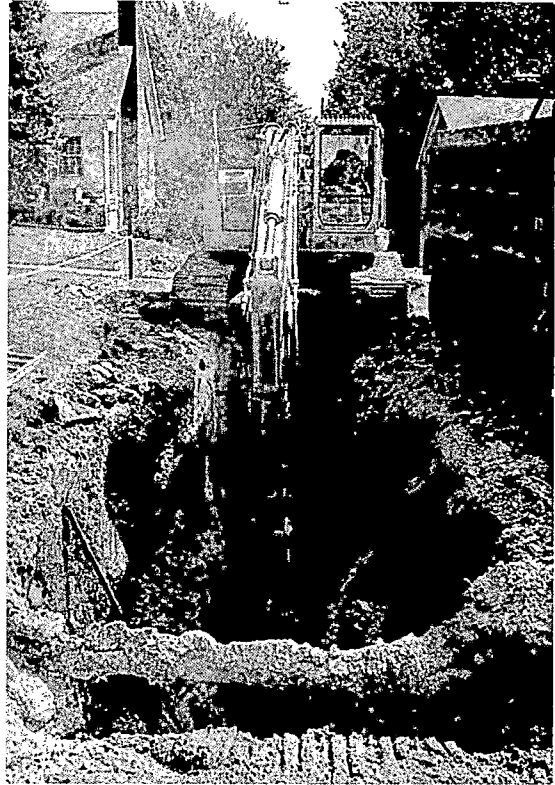
Stantec capitalized on realignment opportunities in the design of the Elkhorn Park trunk sewer replacement to reduce construction costs and minimize disruption to residents in this mature neighborhood.
