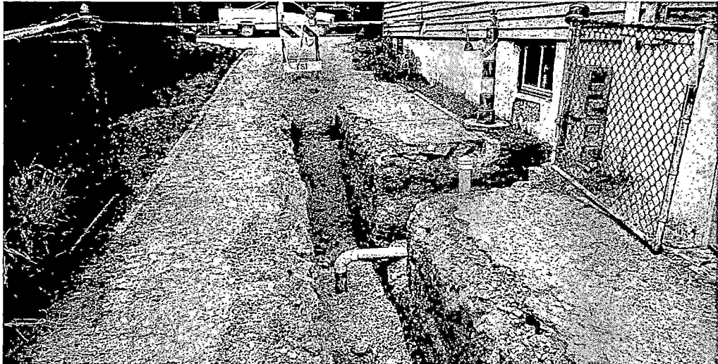
Relocation of Louisville MSD's sewer from the backyards to the street necessitated reconfiguration and replacement of private sewer laterals.
