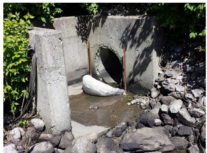
OUTFALL STRUCTURE—120HW (Note staining on rock channel)
