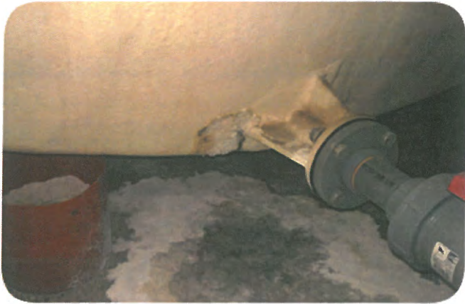
Leak at storage tank drain
