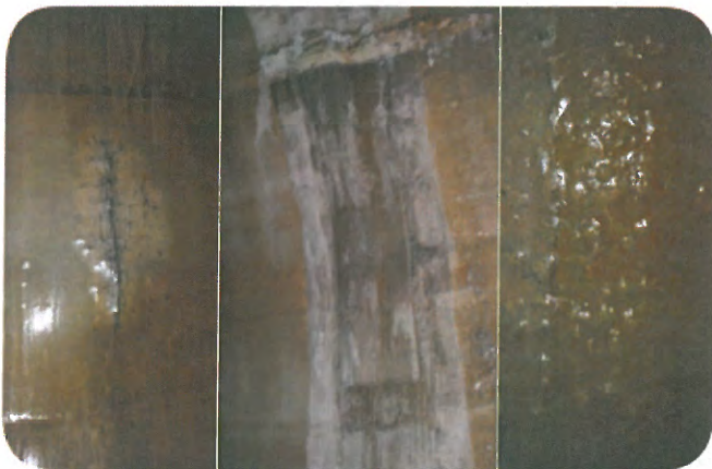
Severe corrosion to storage tank interior – sample close-ups of 3 locations
