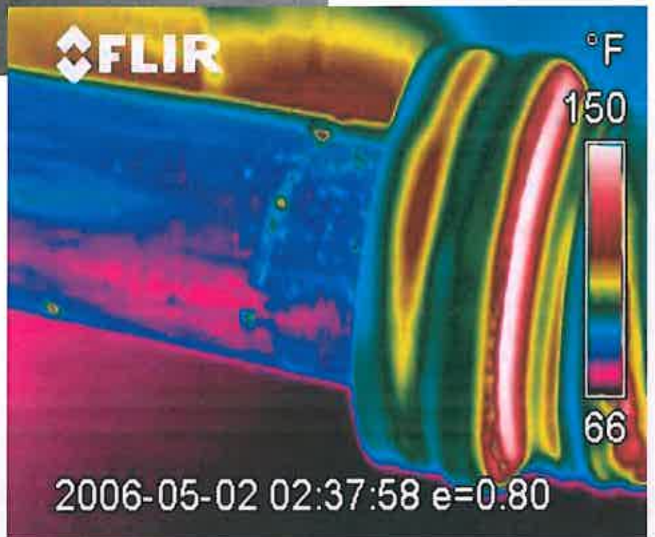
Nozzle leakage- temperature
