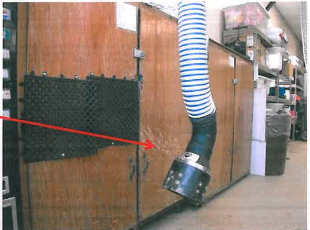
DAMAGE TO CABINETS FROM SWINGING HOSE & NOZZLE
