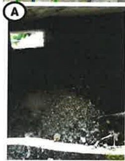
A Sediment has accumulated downstream at the Beacon Hill Road culverts, restricting flow capacity.
