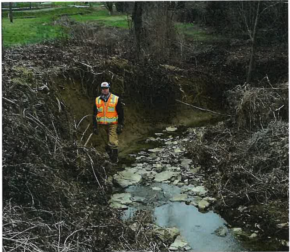
Stantec and Ridgewater have completed nearly 30 projects over the past decade, largely focused in Fayette County. Eric Dawalt (Ridgewater's President) completed the 2020 Feasibility Study with Stantec.
