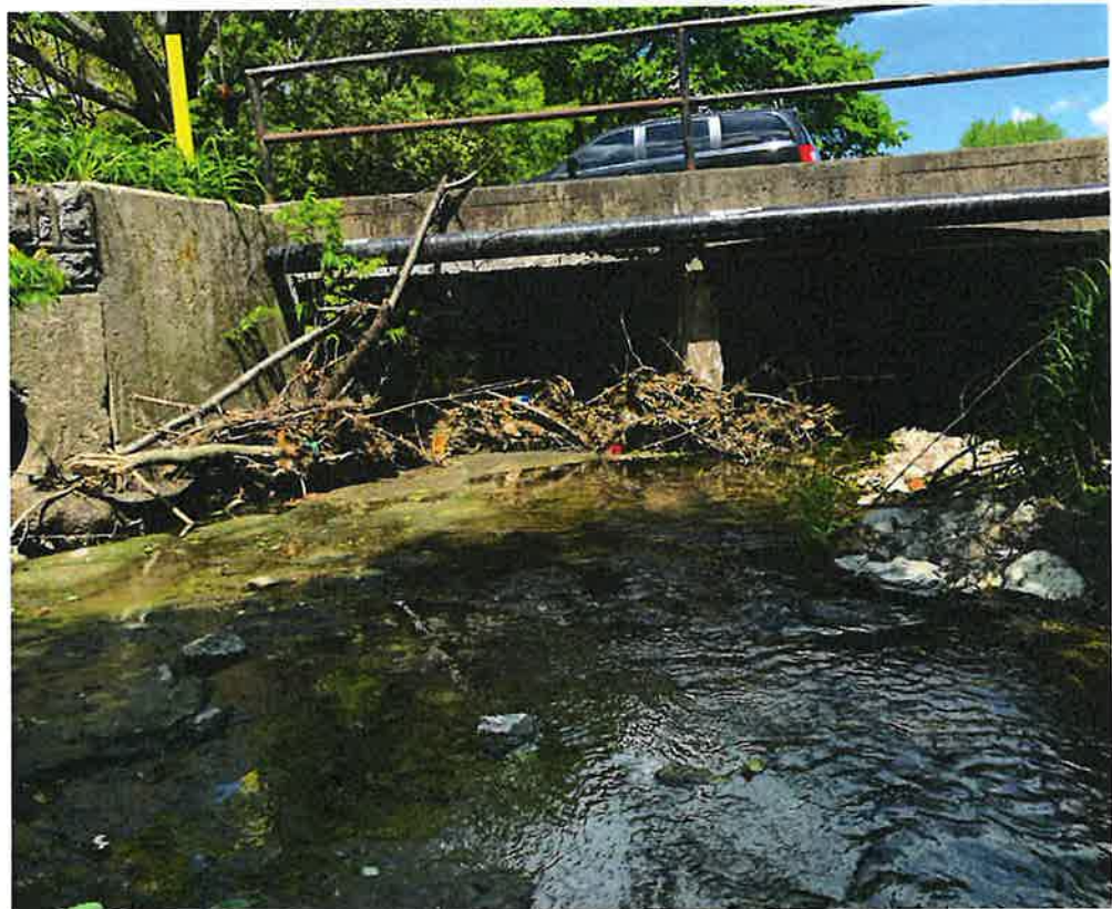
Wolf Run flowing underneath Bescon Hill Road. Stantec's design will evaluate options to reduce the extensive amount of gross debris collecting under the road (and attributing to upstream flooding from the reduced flow capacity).
