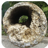
Pipe clogged with FOG
