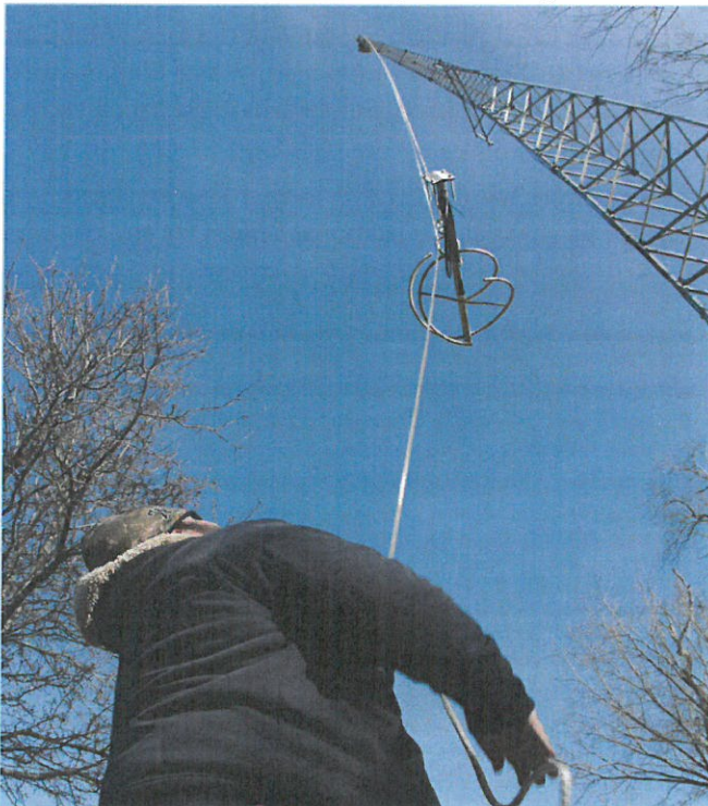
William Willhoite of Antennas Unlimited hoists LCR's transmitter antenna to fellow employee Stephen Barrett, atop the tower. photo: Mick Jeffries
