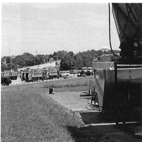
Figure 4.1: Landfill Gas Management System Vent
