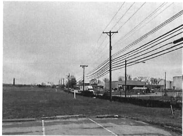
Overhead utilities along Old Frankfort Pike.
