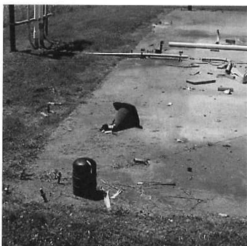
Figure 4.2: Landfill Gas Management System Vent
