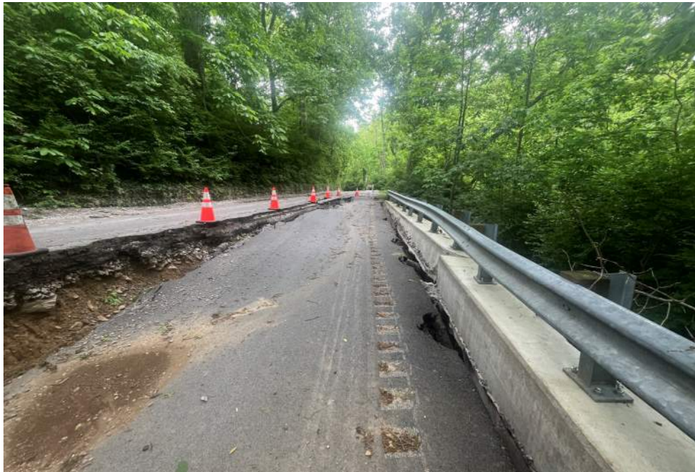
FIGURE 2 - TYPICAL VIEW OF FAILURE (LOOKING SOUTH)
