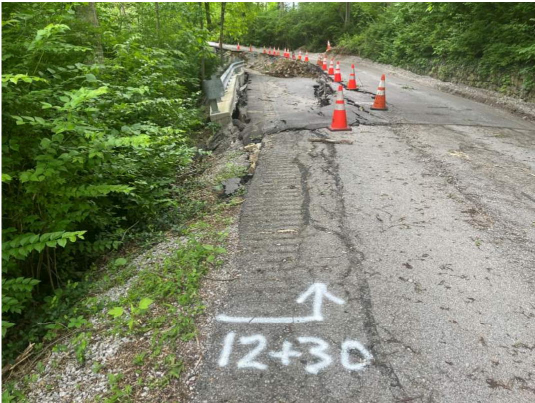
FIGURE 1 - TYPICAL VIEW OF FAILURE (SOUTH END)
