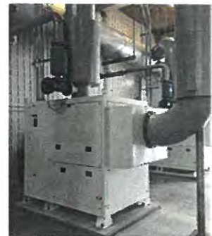
Waukesha high-speed aeration blowers.
