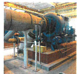
Existing 1,250 HP Roots Blower
