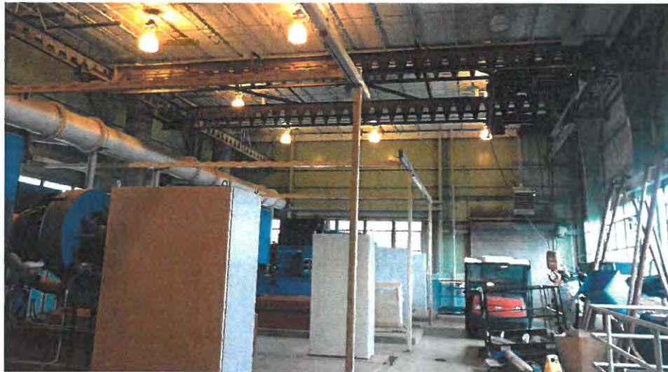
Existing Blower Room at Town Branch WWTP
