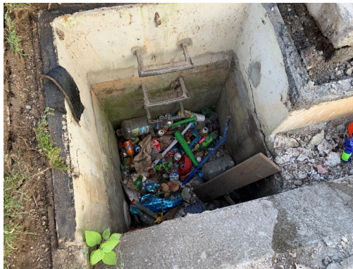
Curb Inlets full of Trash
