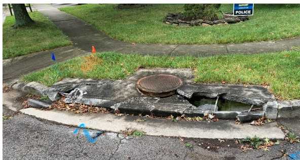
Completely Broken Inlets
