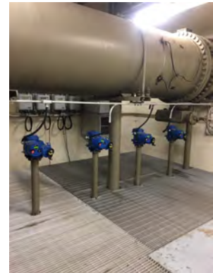
Pump station discharge pipe to aeration influent.
