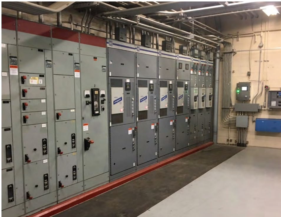
Existing motor control center and variable frequency drives to be replaced.
