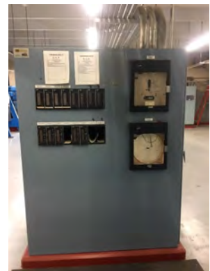
Existing motor panel.
