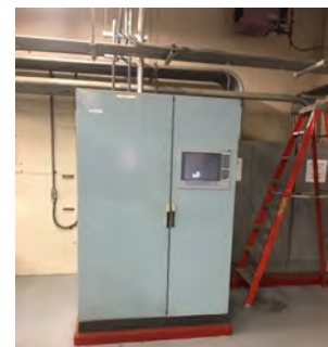
DCU upgraded in recent SCADA replacement project.
