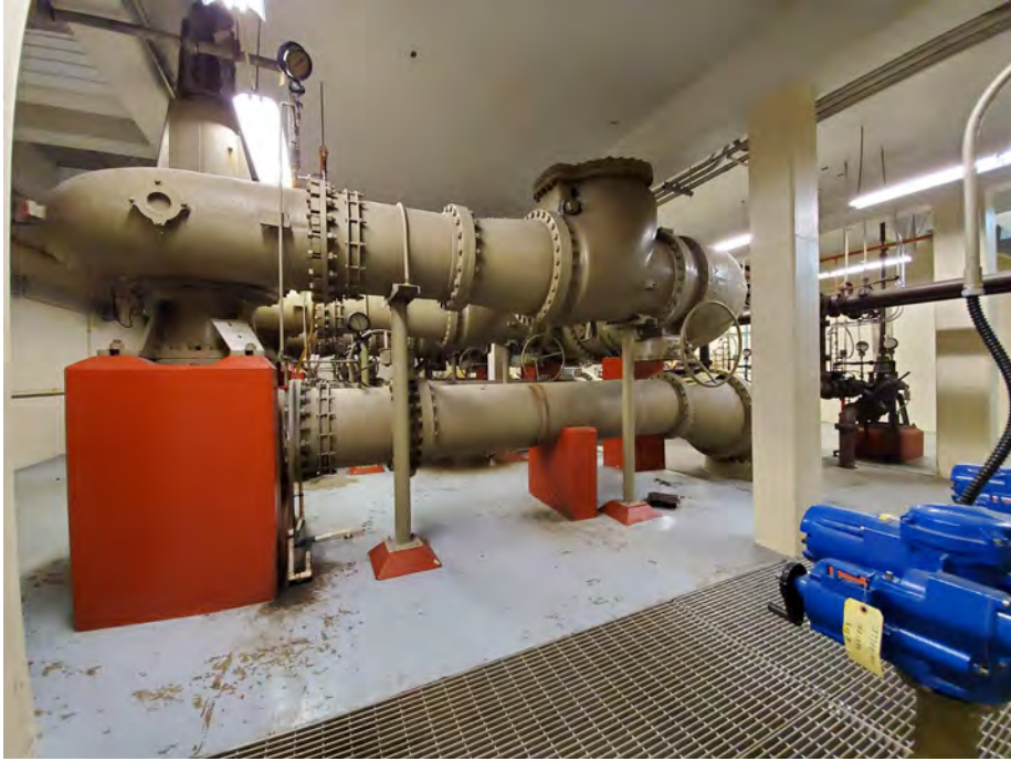
GENERAL PHOTO OF THE AREA AND PIPING
