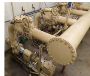
Existing drain pumping station dry well with pumps.
