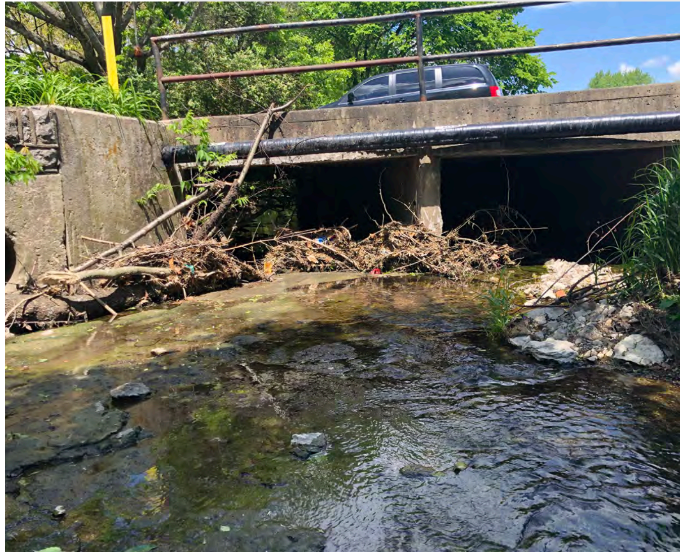
Wolf Run flowing underneath Beacon Hill Road. Stantec's design will evaluate options to reduce the extensive amount of gross debris collecting under the road (and attributing to upstream flooding from the reduced flow capacity).
