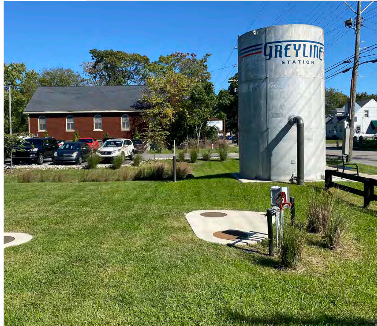
Greyline Station Rainwater Harvest System - completed with a FY2020 LFUCG Stormwater Quality Projects Incentive Grant (Designed/Built by the Stantec/Ridgewater Team). Project was recognized with the 2021 ACEC Grand Award.
