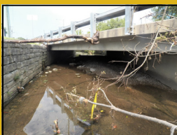
Dead storage within the structure along Manchester Rd., the location of the log indication the depth of water during a storm event. Structure crosses Town Branch with high skew angle.
