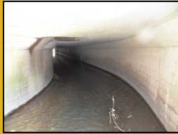
Curvature within the culvert at Cox Street, approximately 600 LF downstream of Begin of Study area.
