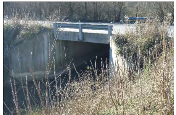
Existing bridge restricts flow at property limit.
