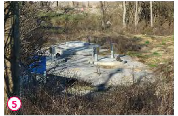
5 New Pump Station
