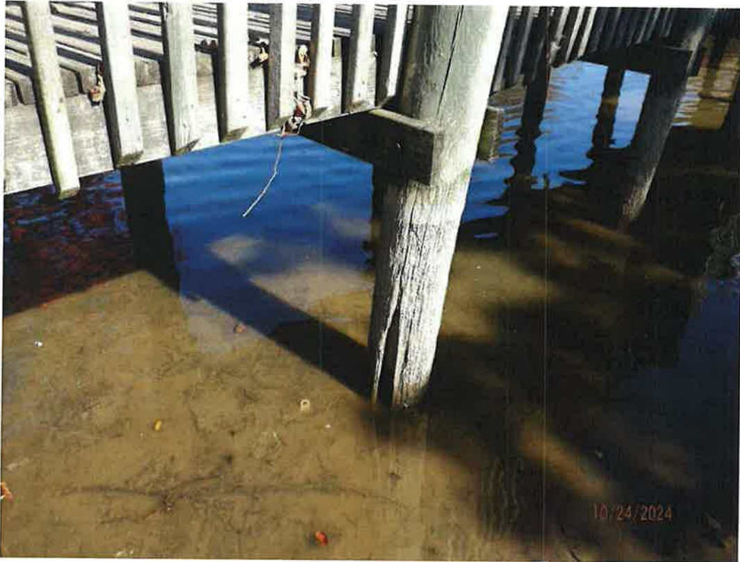
Typical Cavity where a Portion of the Pile has Broken Off. Note Reduction in Circumference near the waterline.
