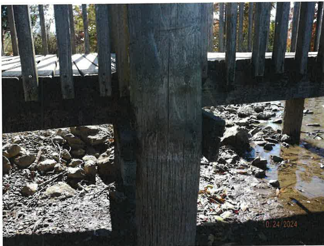
Sounding with Hammer Indicates Hollow Pile near the Waterline
