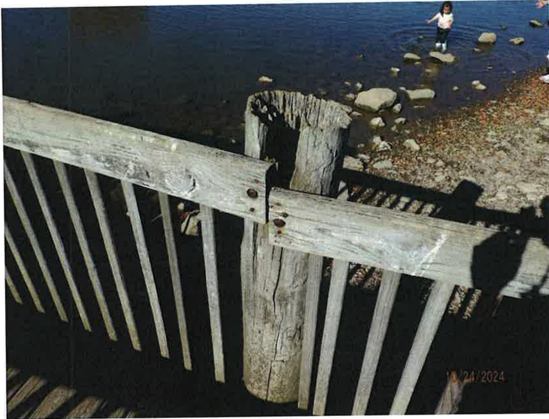
Typical Hollow Pile Top from Deterioration.
