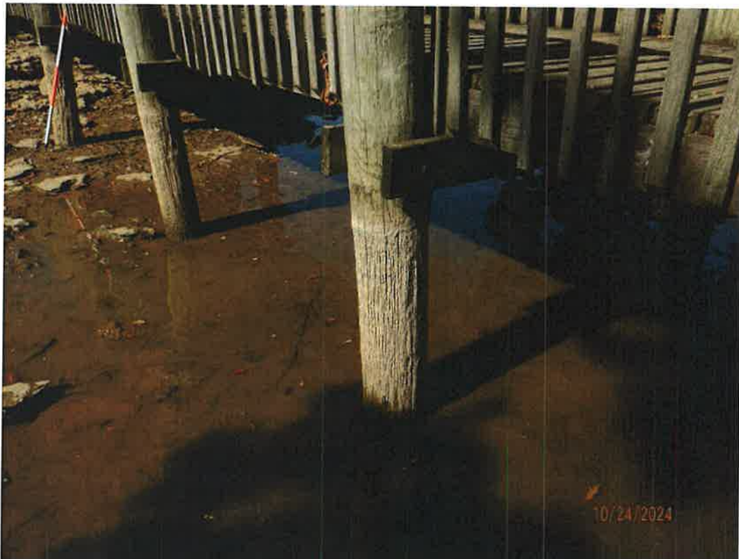
Typical Pile Wear
