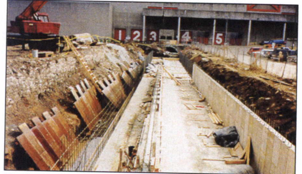
Heritage Hall Expansion - Chambered 12-foot x 6-foot storm and 5-foot x 4-foot sanitary R.C. Box Culvert - Upstream Town Branch Creek.
