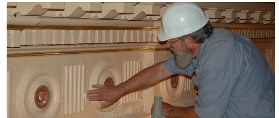
Laylight Over Rotunda Dome Exposure of 1904-1908 Decorative Painting Decorative Stencil in Senate Chamber Revealed Examining the Existing Decorative Interior Plaster for Water Damage Exposure of Paint on Canvas Glued to the Plaster Wall in House Chambers
