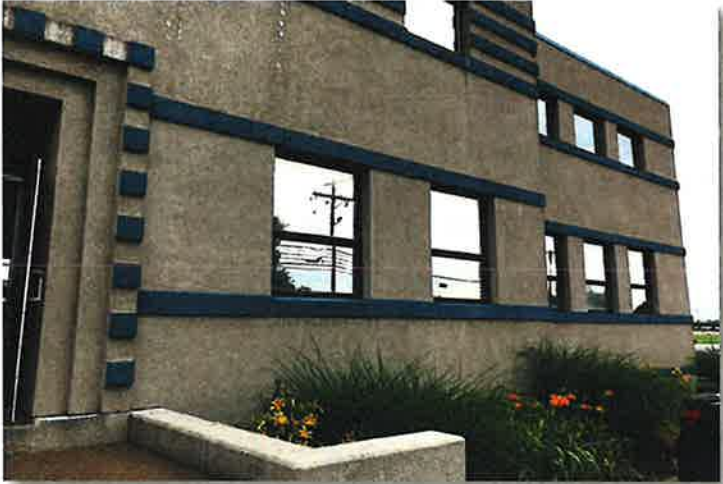
South Façade Condition
