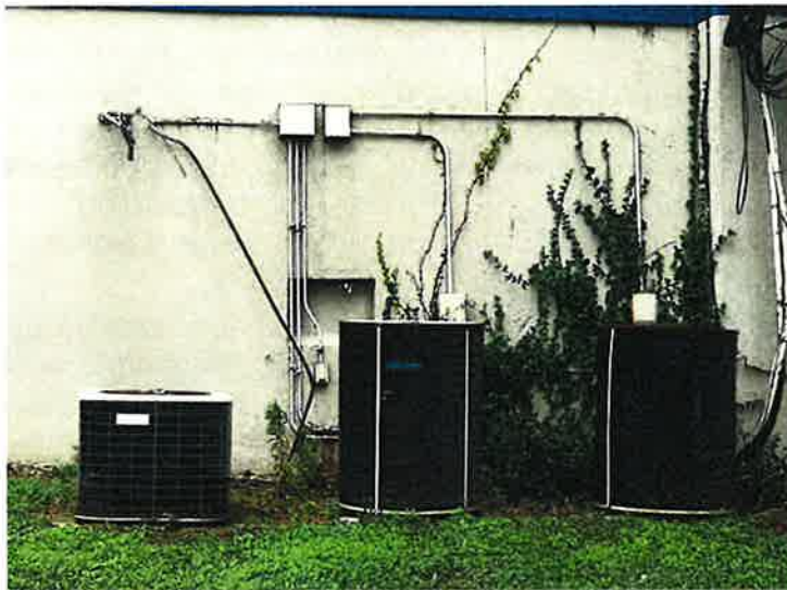
Condensing units and disconnects
