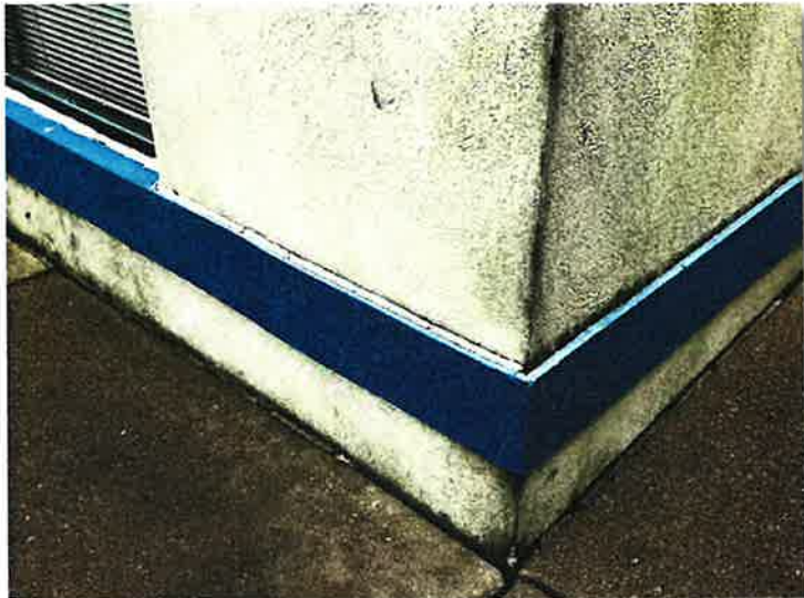
Joint at bottom of EIFS and Sidewalk & Caulk at Window Sill
