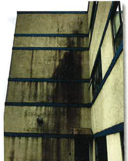
Water Damage at North Stair
