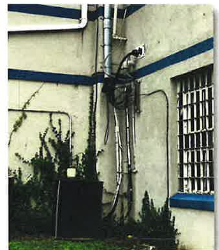
Data, Mechanical & Electrical
