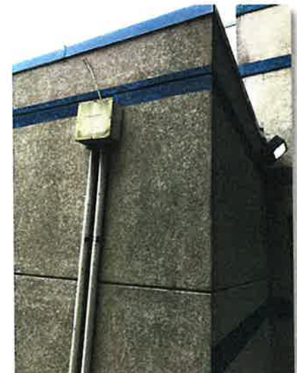
Surface-mounted junction box
