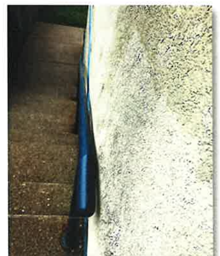
Deformation of Wall at Handrail
