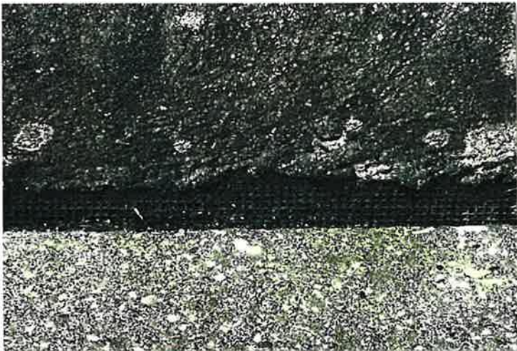
Exposed Reinforcing Mesh at bottom of EIFS
