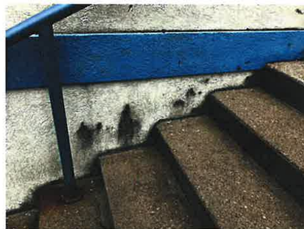
Deterioration of EIFS at the West façade of the West Roll Call Building due to lack of drainage.
