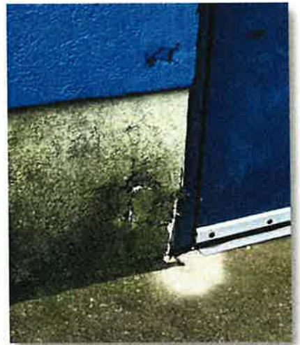
Crushed EIFS at Stair Door
