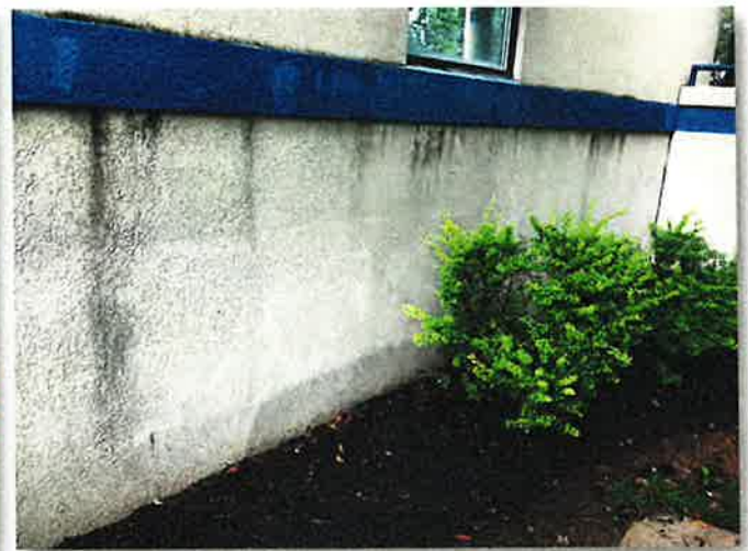
Deformations in EIFS at bottom of wall – Terminates at grade
