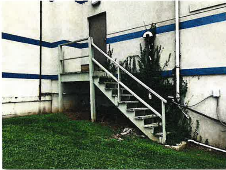
Wood egress stairs over gas service
