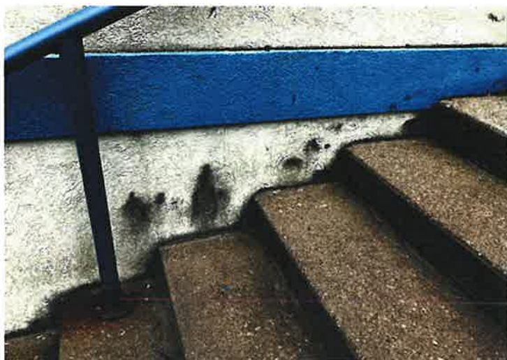
Deterioration of EIFS at bottom of West Façade
