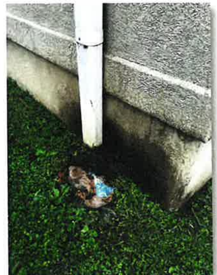
Downspout with no splash block
