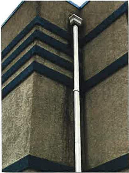
Water damage at poorly functioning scuppers.
