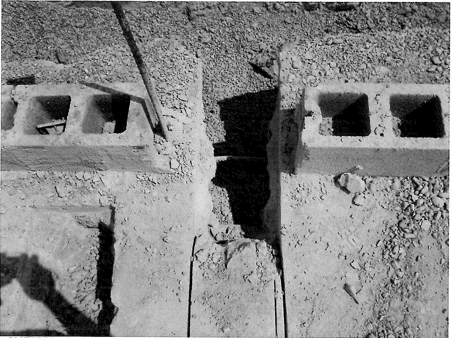
FOOTING BREACHED TO SUB-GRADE 12" WIDE X 28 INCHES LONG IN AREA A CHASE AS SHOWN ON PREVIOUS PAGE
