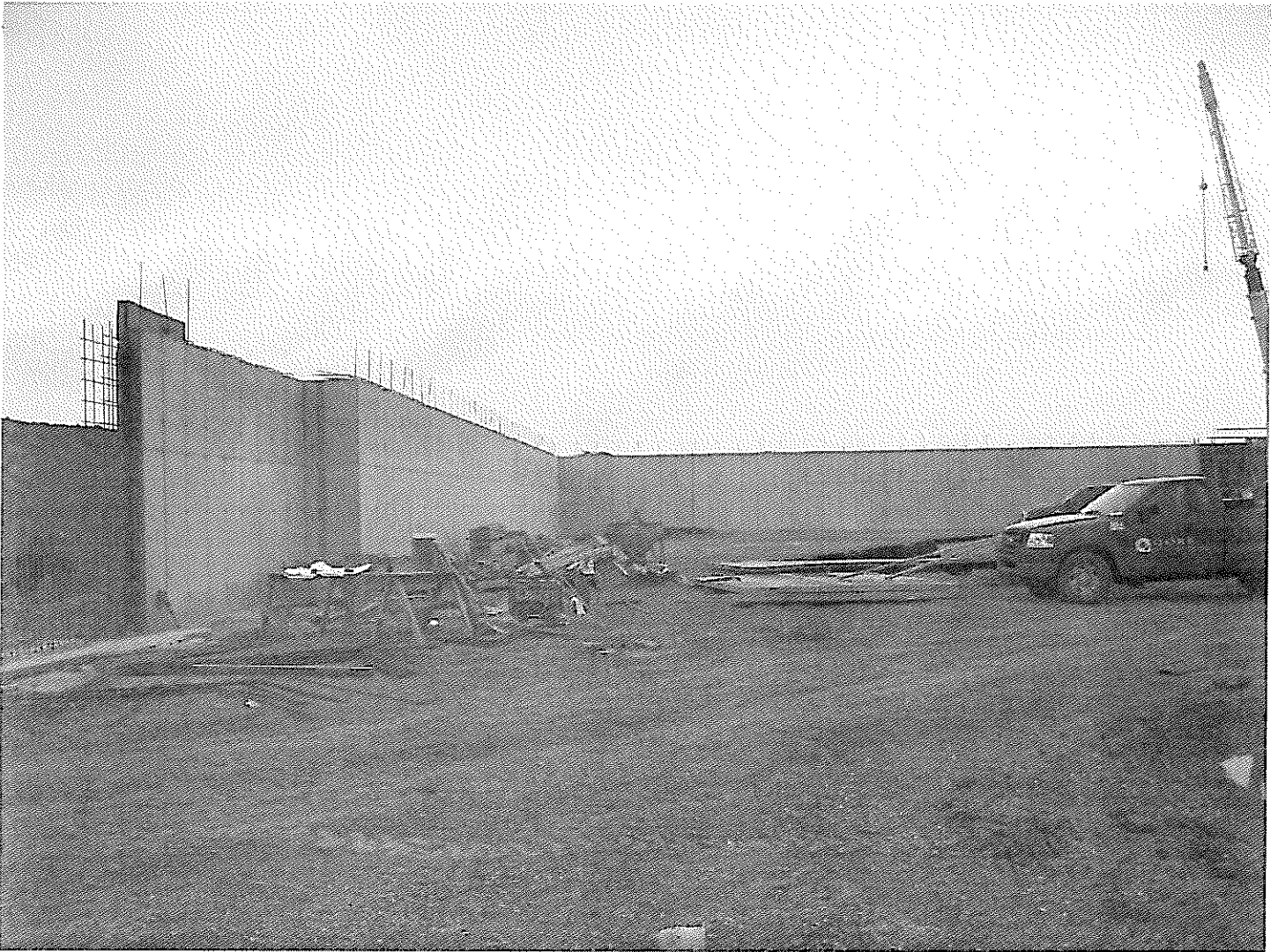
AREA A / AREA B RETAINING WALL FACE WHICH DOES NOT DISPLAY HONEYCOMBING, CRACKING, OR FINS
