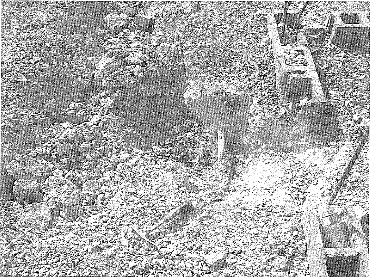
INTERIOR LOAD BEARING FOOTING BREACHED TO SUB-GRADE 28 INCHES WIDE 1 FOOT EAST OF DOORWAY TO RESTROOMS 116 AND 117
