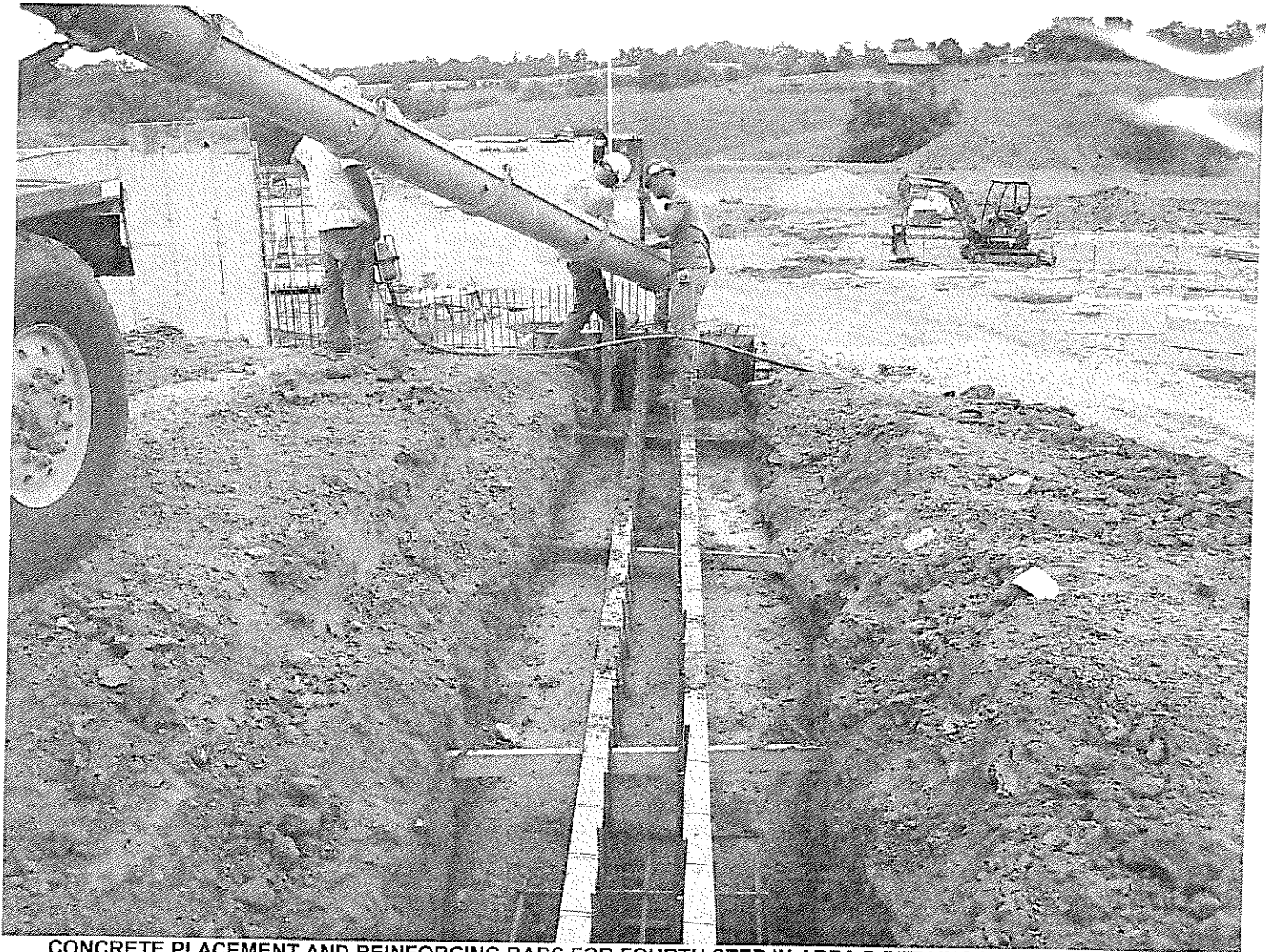
CONCRETE PLACEMENT AND REINFORCING BARS FOR FOURTH STEP IN AREA B RETAINING WALL @ MATCHLINE
