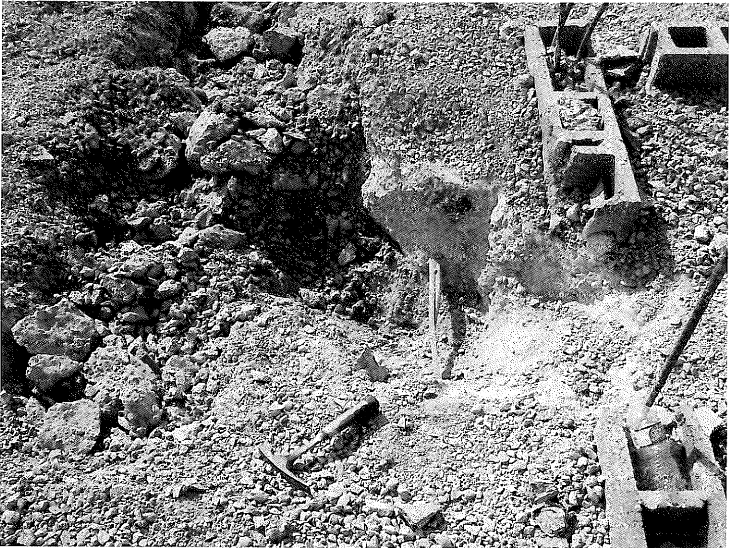
INTERIOR LOAD BEARING FOOTING BREACHED TO SUB-GRADE 28 INCHES WIDE 1 FOOT EAST OF DOORWAY TO RESTROOMS 116 AND 117
