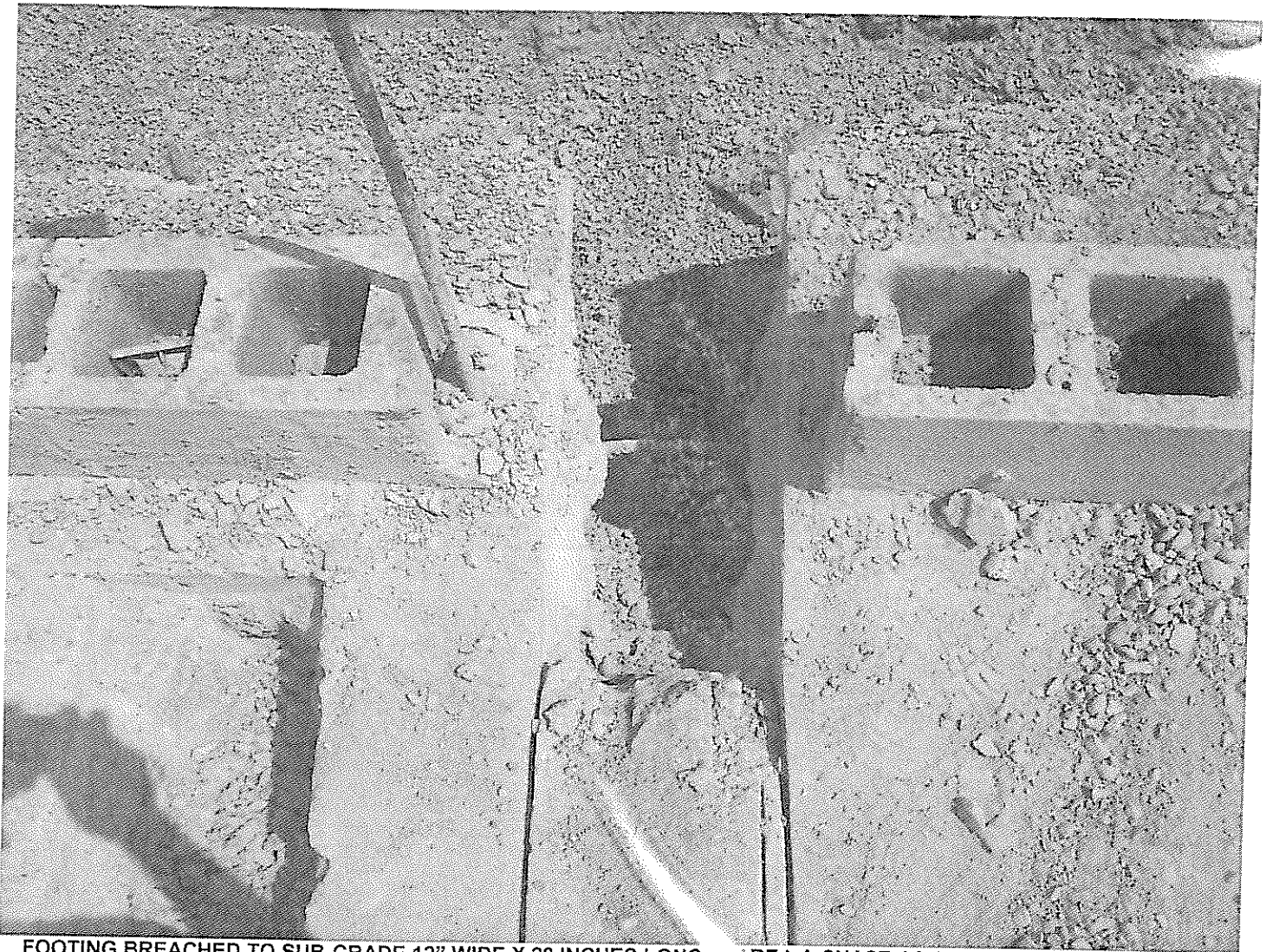
FOOTING BREACHED TO SUB-GRADE 12" WIDE X 28 INCHES LONG. AREA A CHASE AS SHOWN ON PREVIOUS PAGE
