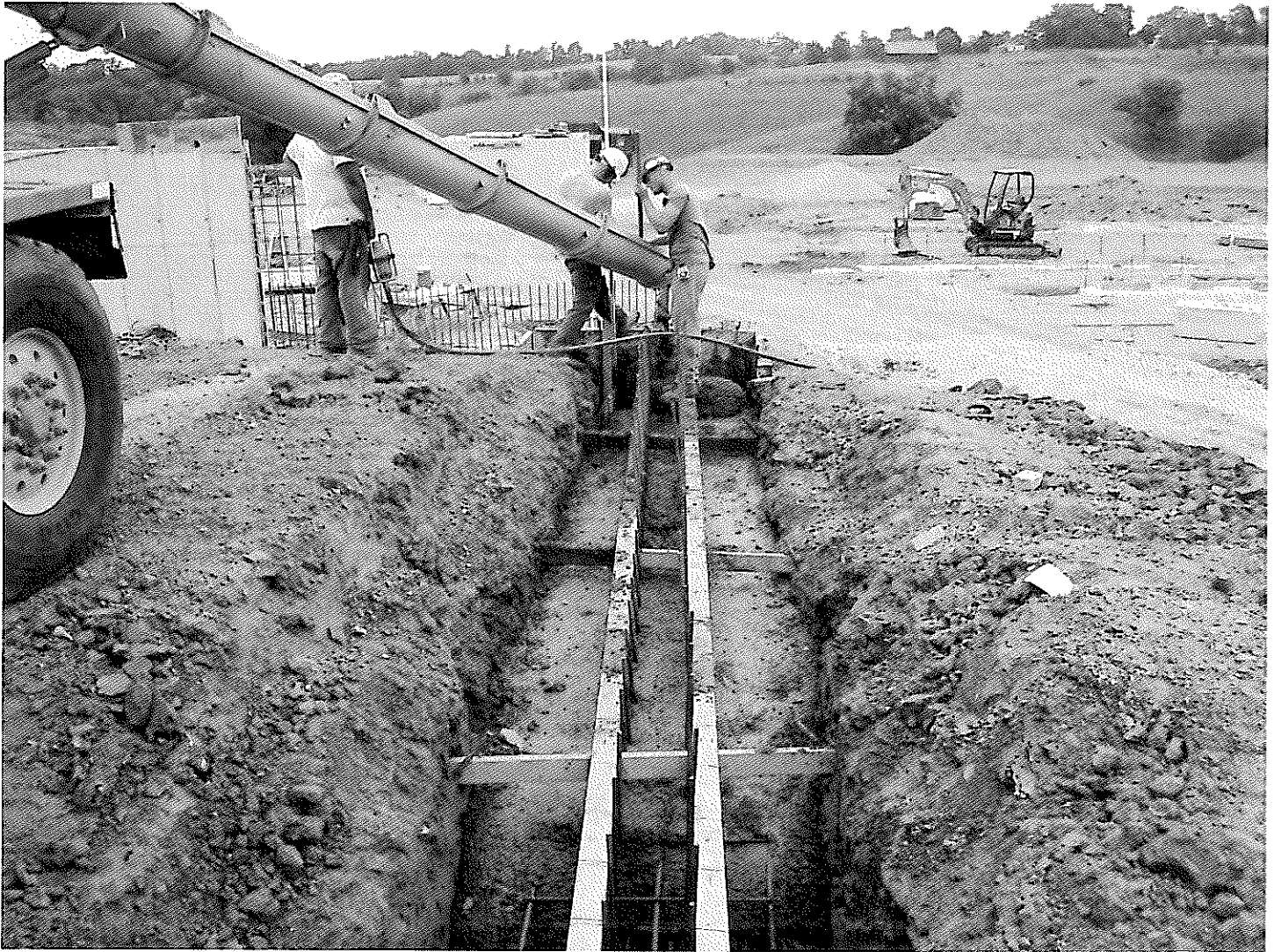
CONCRETE PLACEMENT AND REINFORCING BARS FOR FOURTH STEP IN AREA B RETAINING WALL @ MATCHLINE
