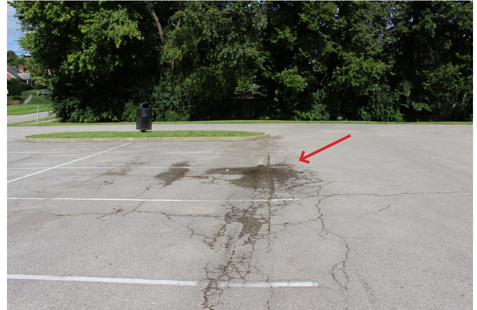
FIGURE #5: examples of multiple cracks that needs further evaluation for more in-depth repairs & early stages of pothole formation (pointed out in red)
