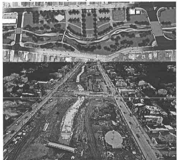
Lick Run Valley Conveyance System – Cincinnati, OH. (Ongoing)
