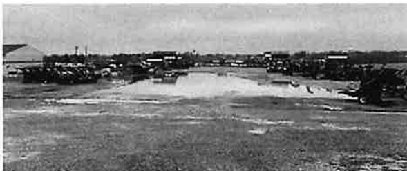
Existing building pad and ponded water.
