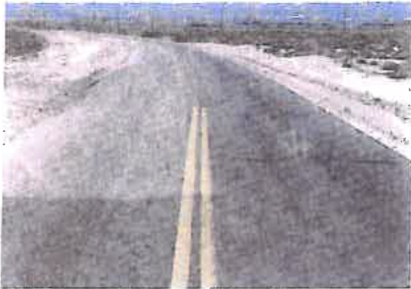
Reclamite was used as a construction seal. For comparison, the lower left area was not treated.
