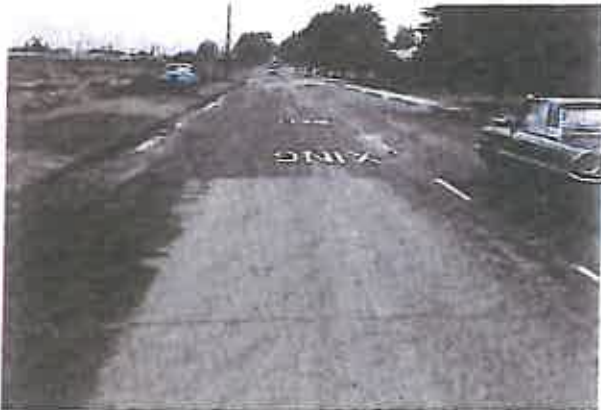
Reclamite was used as a construction seal on the dry areas of this pavement. Untreated areas are still wet from water penetrating the surface.
